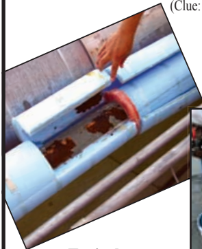
Typical CUI Problem
